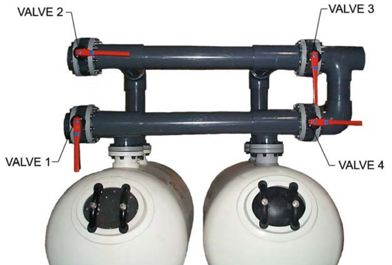
Dual Tank System Piping at Right (Filter Mode)
